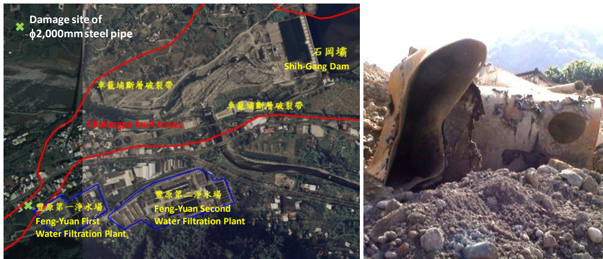
Figure 1 A \phi 2,000\text{mm} steel pipe bent and damaged at Chelungpu fault crossing near the Feng-Yuan First Water Filtration Plant in Chi-Chi earthquake (courtesy Taiwan Water Corp.)
