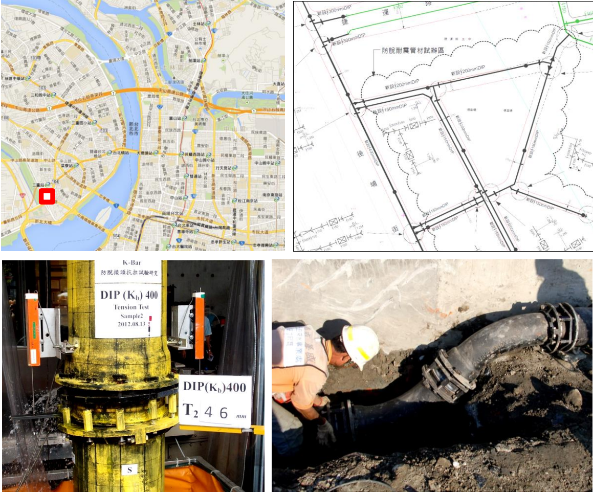
Figure 6 A pilot project using K-bar slip-out resistant ductile iron water pipes in Erchong Floodway Redevelopment Zone, Sanchong, New Taipei city (Wu 2014; courtesy TWD)
