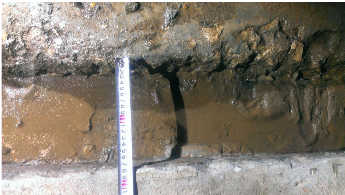
Figure 4 The expansion of the extension joint
