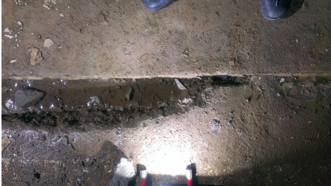
Figure 3 The crack caused by interactional bump of base plate of water tank
