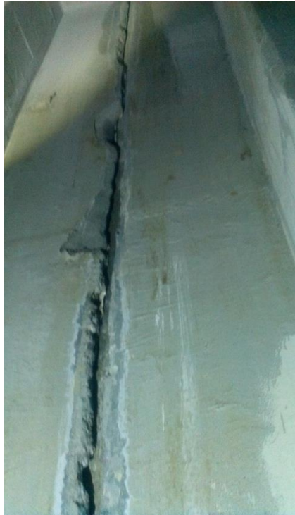
Figure 5 the crack of wall
