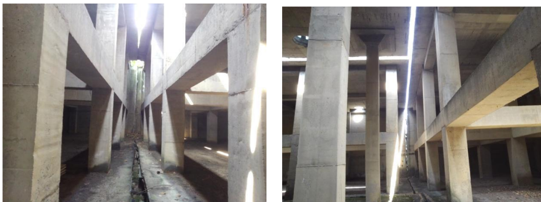
Figure 7 The severe expansion of extension joint
