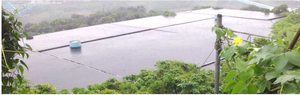
Figure 1 The roof of water tank – the failure of extension joint by expansion
