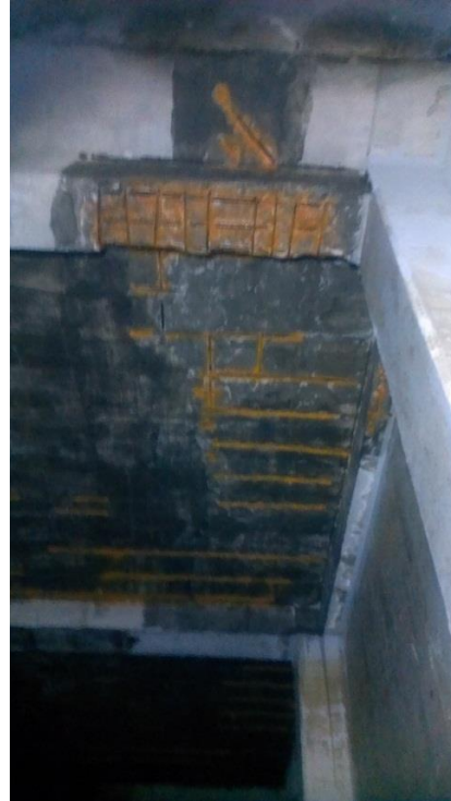
Figure 6 the crack of the joint of beam and column
