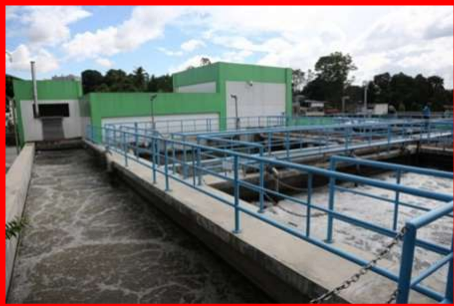
San Antonio and Del Monte STP's
