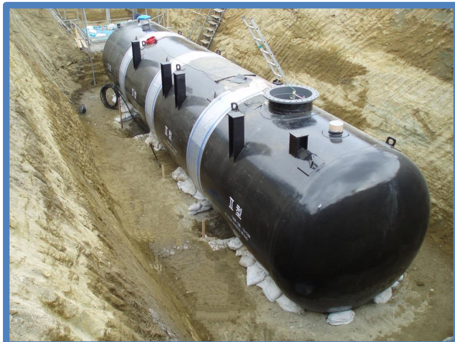
Figure1 - Emergency drinking water storage tank
