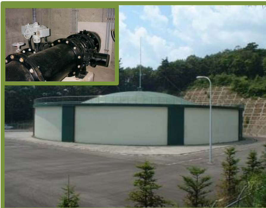
Figure3 - Water reservoir with Emergency stop valves
