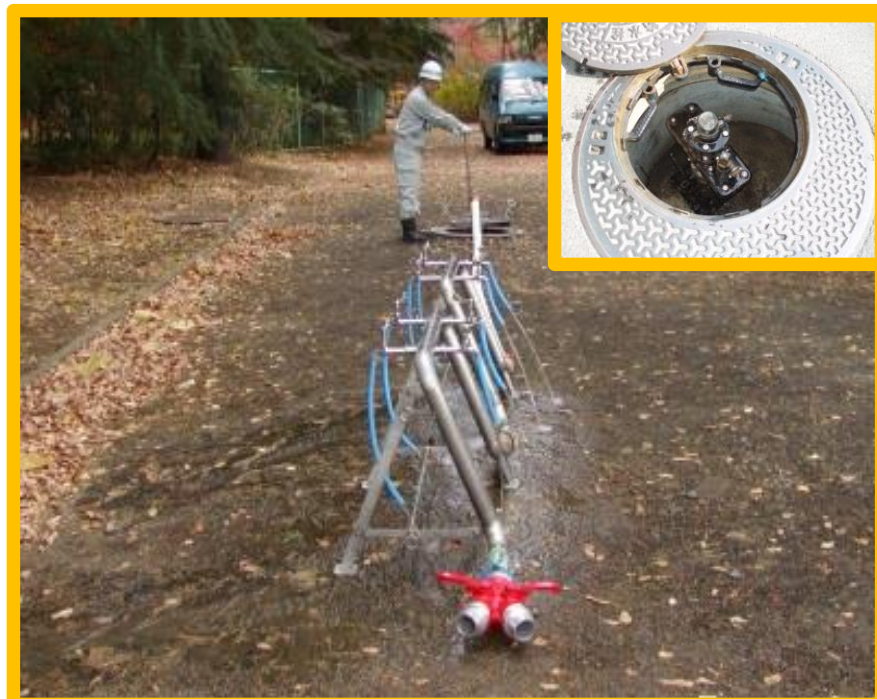
Figure2 - Emergency water supply taps [main pipe type] (24 locations)
