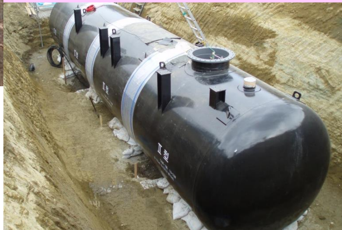
Emergency drinking water storage tank (21 locations)
