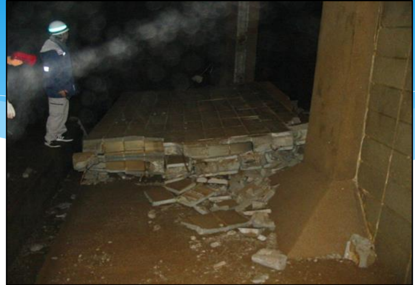
Collapse of flow arrangement wall(Anyoji Reservoir)
