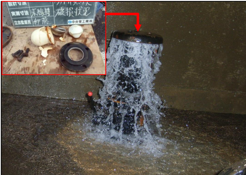
Damage to Air valves on distribution main
