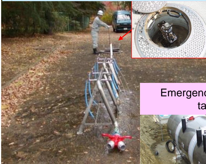
Emergency water supply taps [main pipe type] (24 locations)
