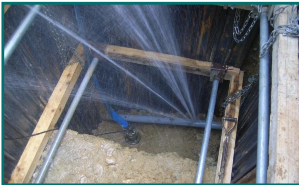
Broken in PVC
